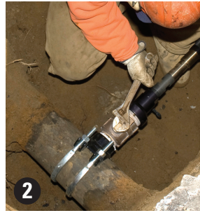
2 Open corp stop valve.
