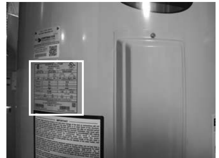
Figure 23 - The water heater’s electrical requirements can be determined from the data plate.
