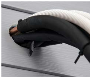
Without a wall sleeve, the insulation and drain hose is easily damaged
