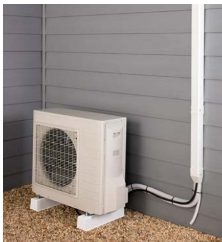
Starter Kit Installed
